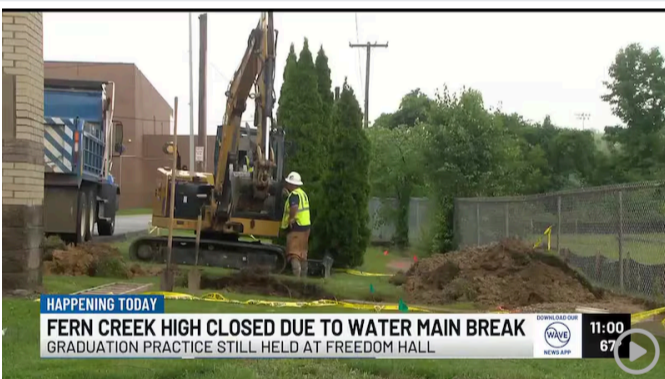
Fern Creek High School cancels classes due to water pipe break
